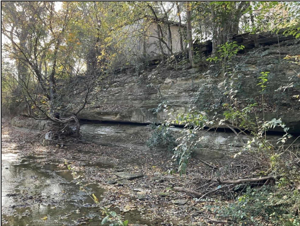
Photo 15 – STA 13+50 – This bank exhibits a “Low” BEHI rating – although the bank is steep, it is composed of bedrock that reduces the overall bank erosion potential.
