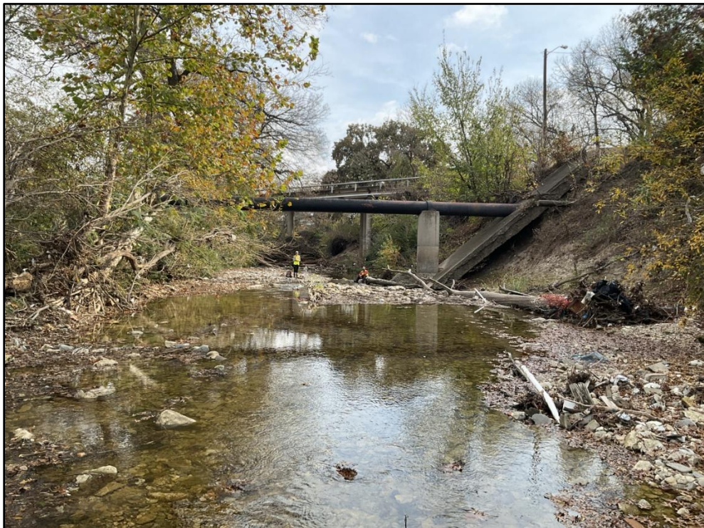
Photo 112 – STA 97+00 – 36-inch aerial sanitary sewer crossing, looking downstream. Right bank protection is undermined.
