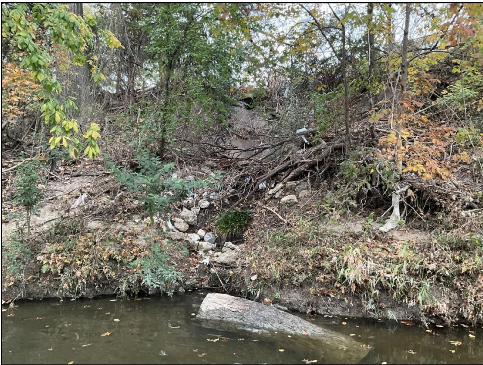
Photo 60 – STA 5+00 – Problem area rank: 16. 18-inch corrugated plastic stormwater outfall with small concrete flume and rock riprap, approximately 6 to 8 feet above the water surface.
