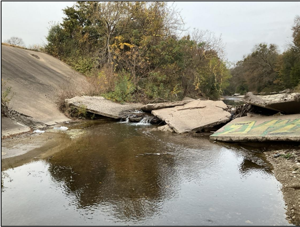
Photo 55 – Near STA 0+00 – Conditions at South Main Street, looking upstream at broken concrete protection in channel.
