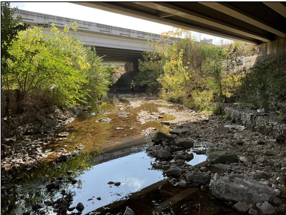
Photo 34 – STA 38+00 – Looking downstream at conditions under Highway 67.
