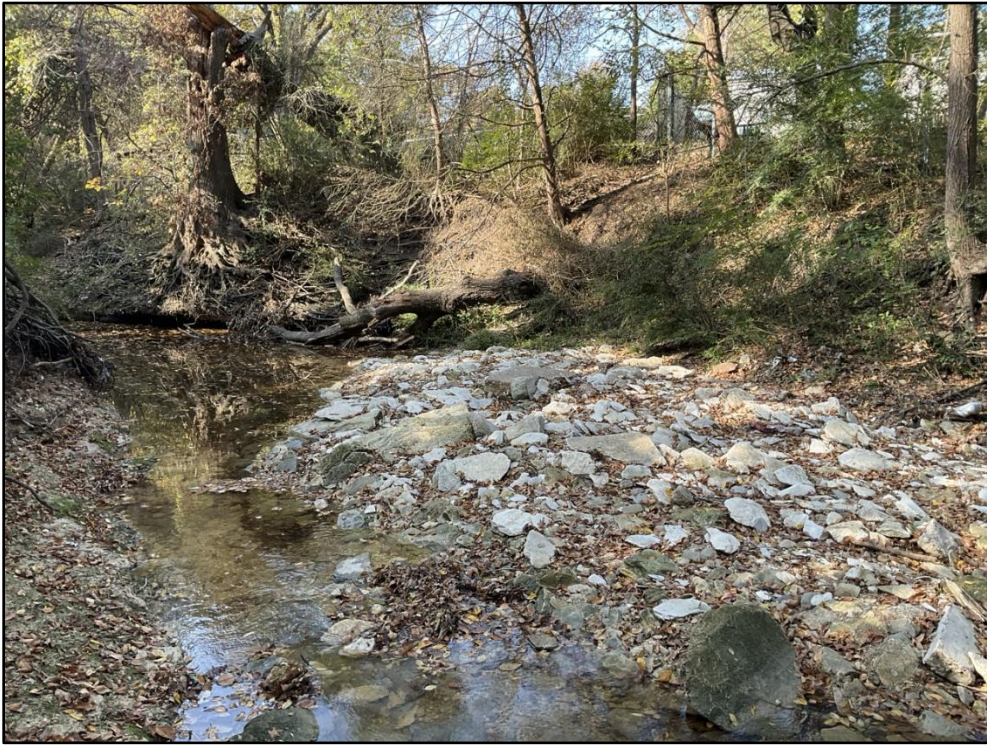
Photo 19 – STA 22+00 – Looking downstream at channel bar composed of broken bedrock and concrete debris. Large broken tree downstream as well.
