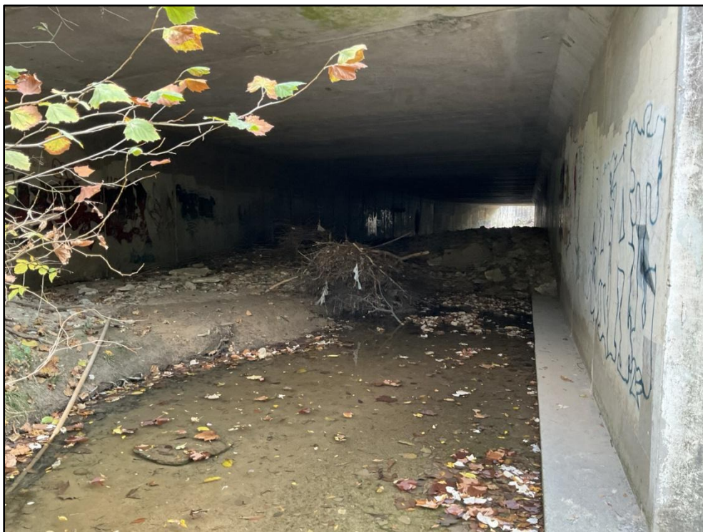
Photo 52 – STA 66+00 – Significant deposition in left cell of East Danieldale Road culvert.
