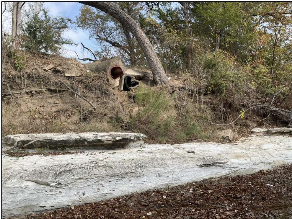
Photo 90 – STA 58+00 – Problem area rank: 18 . Unmapped, likely abandoned pipes protruding from the left bank.
