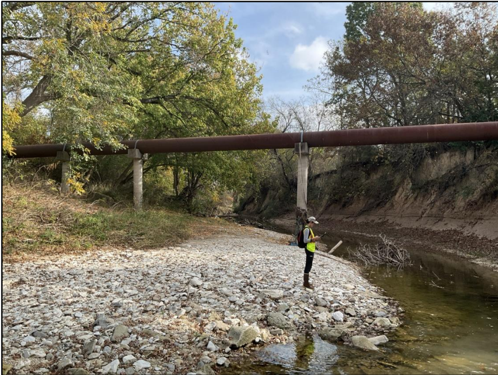
Photo 85 – STA 50+50 – Looking downstream at a 36-inch aerial sanitary sewer crossing. Some piers on left bank appear to be leaning. See Photo 86 for right bank condition.
