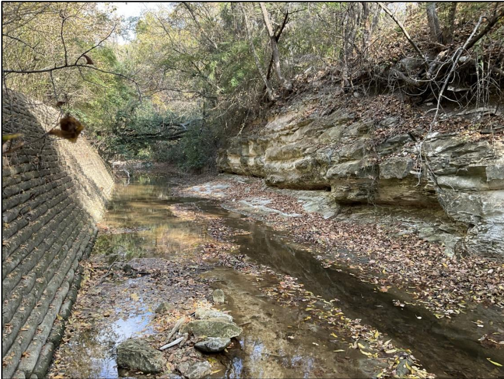
Photo 27 – STA 30+00 – Looking upstream. The channel corridor narrows between Sta. 29+00 – 30+50 where the channel is confined by a concrete bag wall on the right bank and bedrock on the left bank.
