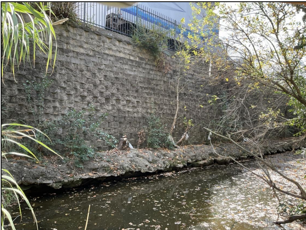
Photo 30 – Near STA 34+00 – Problem area rank: 14 . Modular articulated block wall in poor condition. Grouted riprap toe is undercut by roughly two feet.
