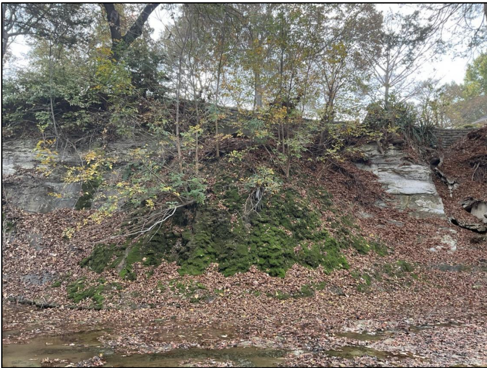
Photo 106 – STA 88+00 – 48-inch concrete stormwater outfall on right bank with patch of moss below.
