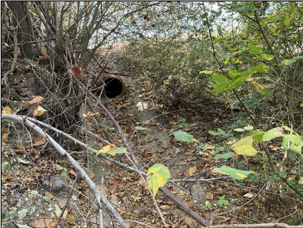
Photo 37 – STA 40+50 – 18-inch concrete stormwater outfall with flume.
