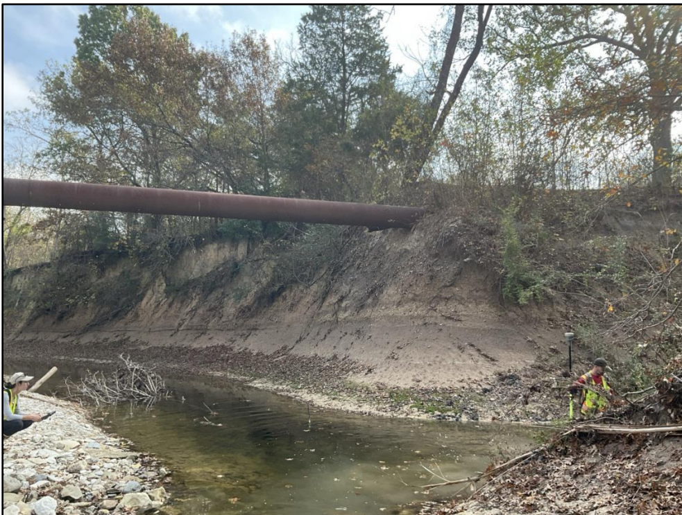
Photo 86 – STA 50+50 – Problem area rank: 2 . Looking downstream at a 36-inch aerial sanitary sewer crossing (also see Photo 85 ). No visible protection on right bank. The pipe is exposed on the right bank of Stewart Branch (at the right edge of the photo).
