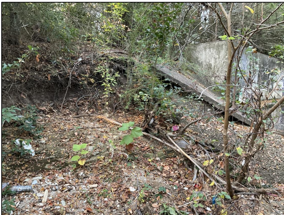
Photo 4 – STA 2+00 – Erosion undermining the downstream end of the concrete head wall.
