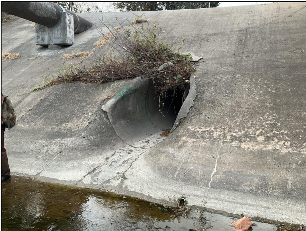
Photo 56 – STA 0+50 – 60-inch concrete stormwater outfall.
