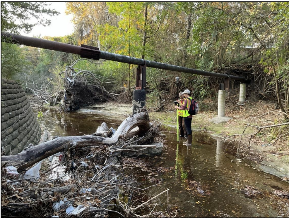
Photo 6 – Near STA 4+50 – Problem area rank: 6 . Private 8-inch utility crossing, looking downstream. Local scour around piers and on right bank.
