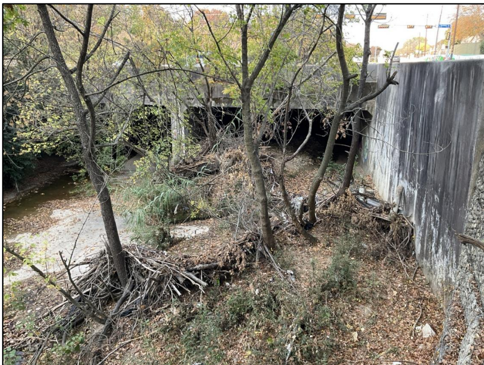
Photo 54 – STA 69+00 – Problem area rank: 20 . Looking upstream at the other side of the East Daniieldale Road culvert. Trees are growing out of well-established sediment deposition in the left cell.
