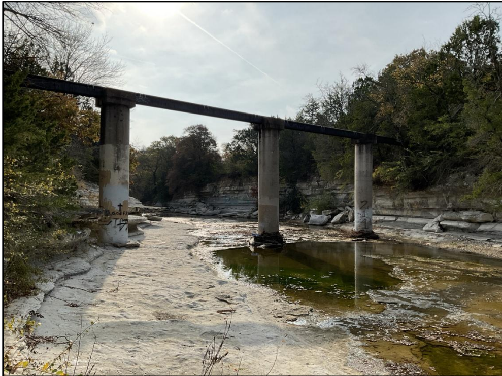
Photo 77 – STA 32+00 – 8-inch aerial sanitary sewer crossing. Minor scour around in-channel piers.
