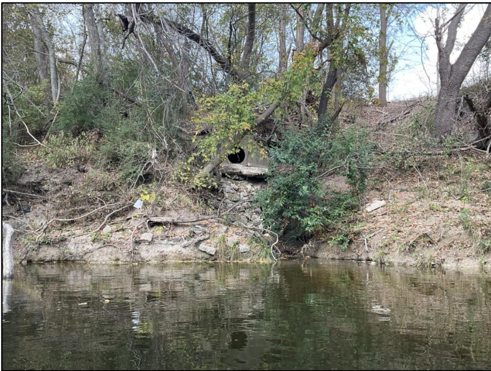
Photo 104 – STA 82+00 – Problem area rank: 19 . Concrete stormwater outfall. Flowline is approximately 8 feet above the water surface.
