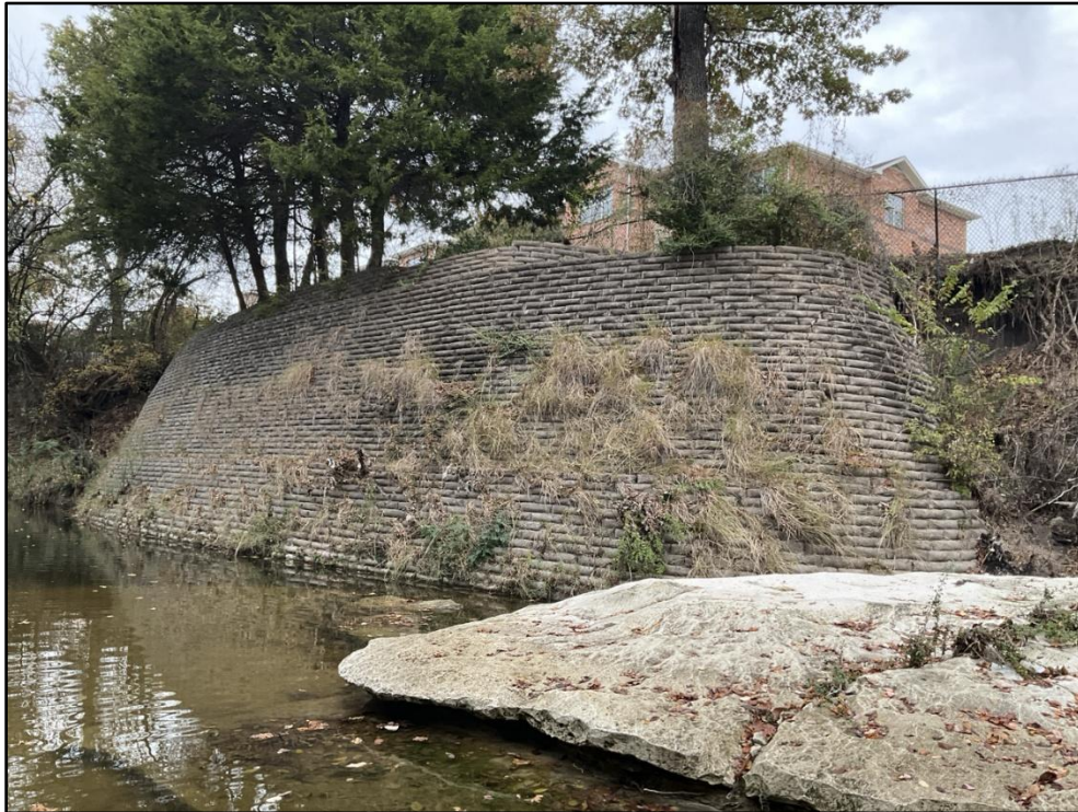
Photo 61 – Near STA 5+50 – Problem area rank: 7 . Concrete bag wall on left bank. There is significant erosion on downstream end of wall and evidence of vertical settling and cracking on the wall.
