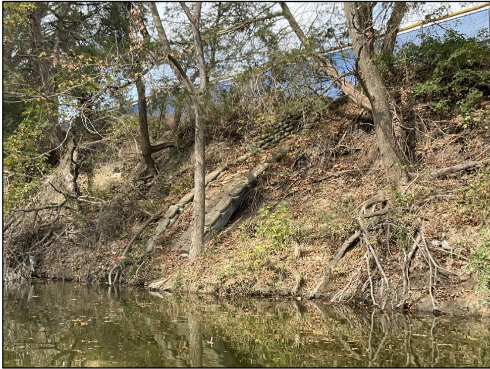
Photo 89 – STA 55+50 – Problem area rank: 17 . Concrete bag wall flume; lower portion is partially undermined.
