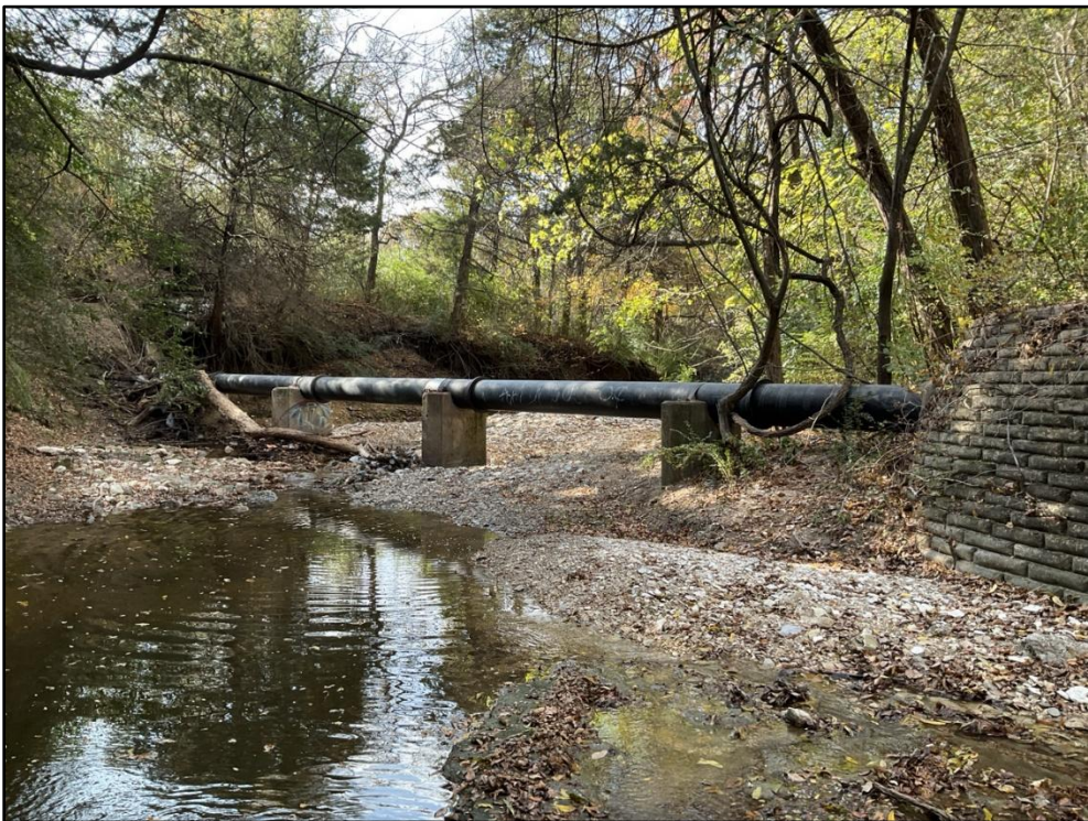
Photo 28 – STA 31+00 – Problem area rank: 4 (★ Area 1 ★) . Looking downstream. A 20-inch sanitary sewer crossing emerges from a bag wall on the right bank. The left bank is heavily eroded around the pipe with no observed protection.
