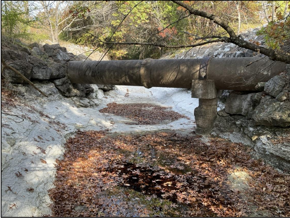
Photo 79 – Near STA 36+50 – Two 36-inch aerial sanitary sewer crossings on Tenmile Creek Unnamed Tributary 5 in fair condition. Moderate deterioration of grouted rock riprap at banks and minor pier scour.
