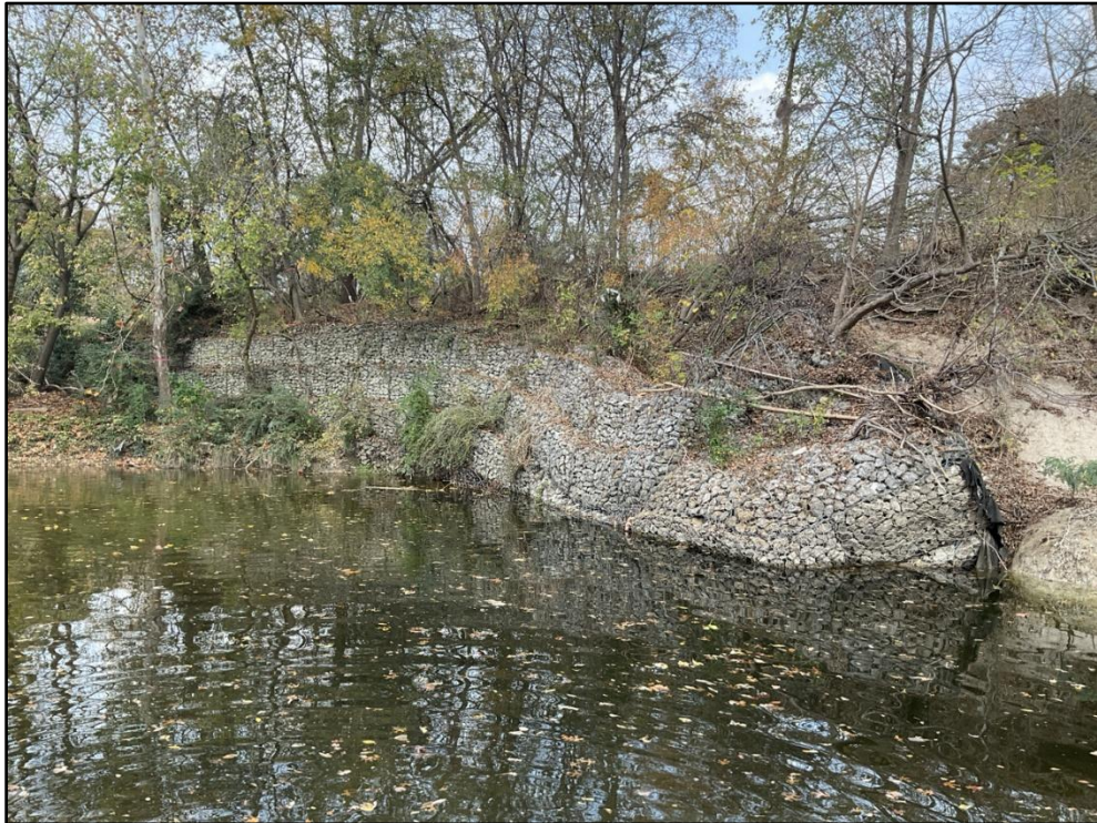
Photo 111 – STA 94+50 – Problem area rank: 3 . Gabion wall along the left bank. The downstream end of the wall has eroded and settled and there is an unmapped exposed pipe.
