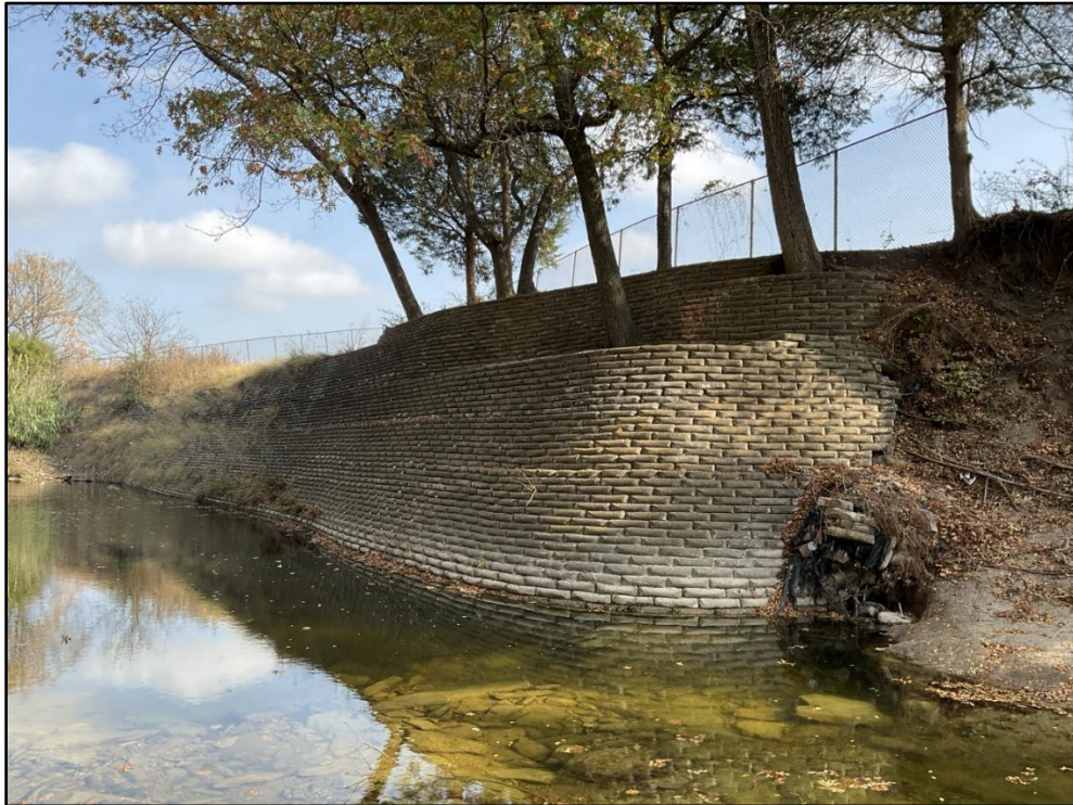
Photo 81 – Near STA 41+00 – Concrete bag wall in fair condition, looking upstream. Some erosion on downstream end and minor toe scour.
