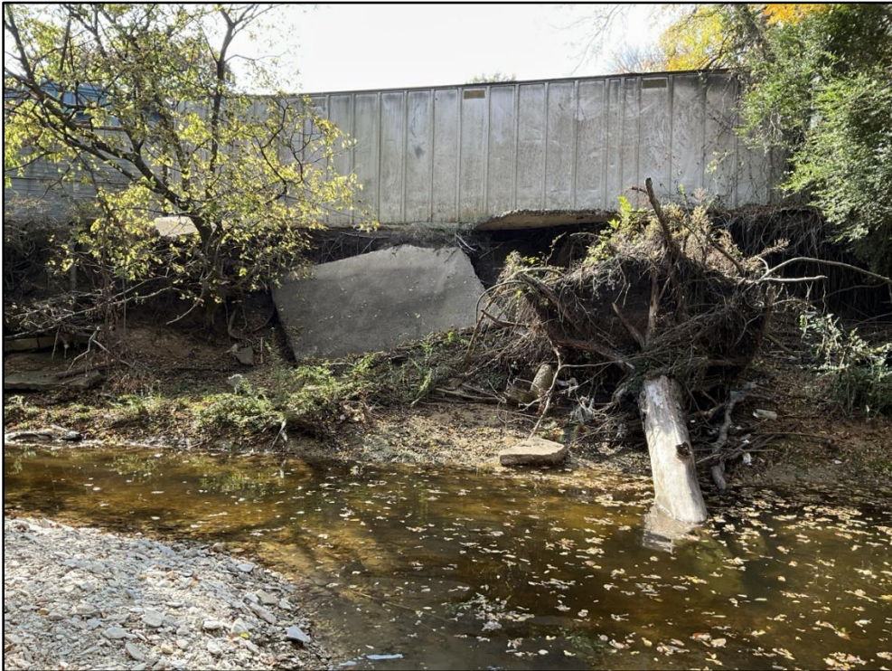
Photo 29 – STA 32+50 – Looking downstream at erosion on outer right bank. Fallen tree and broken concrete protection.
