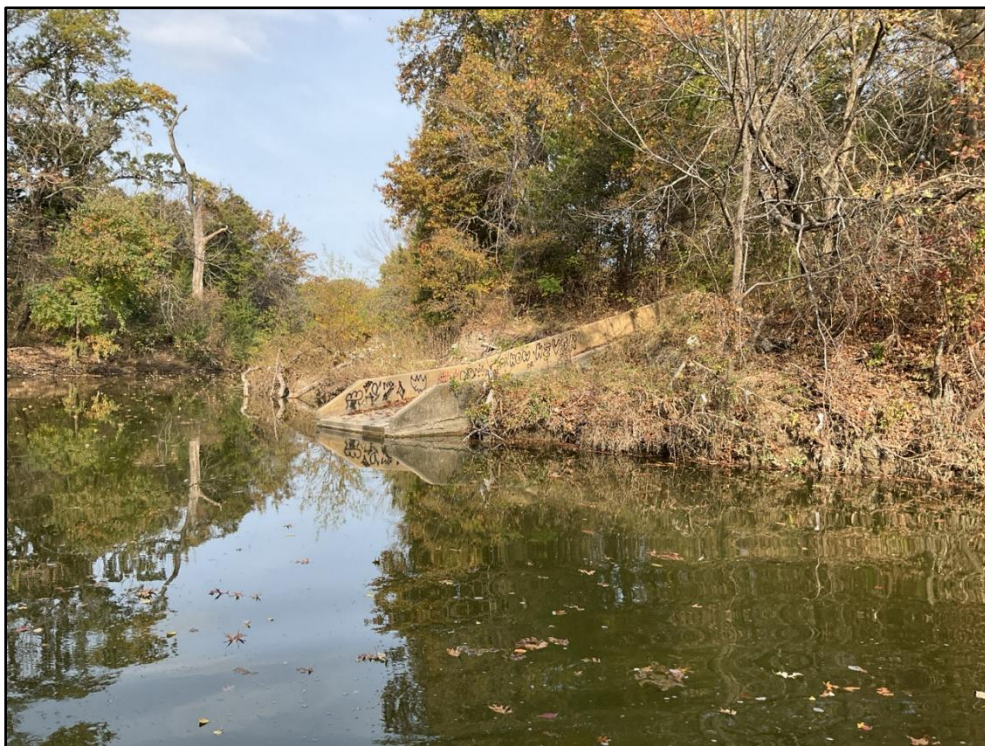
Photo 76 – STA 28+50 – Problem area rank: 11 (★ Area 3 ★) . Looking upstream at a concrete stormwater flume located on a deep scour pool. The flume is undermined and approximately 12 feet above the channel bed elevation.
