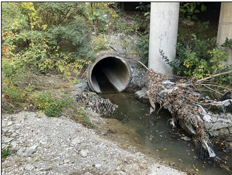
Photo 36 – STA 40+00 – 48-inch concrete stormwater outfall.
