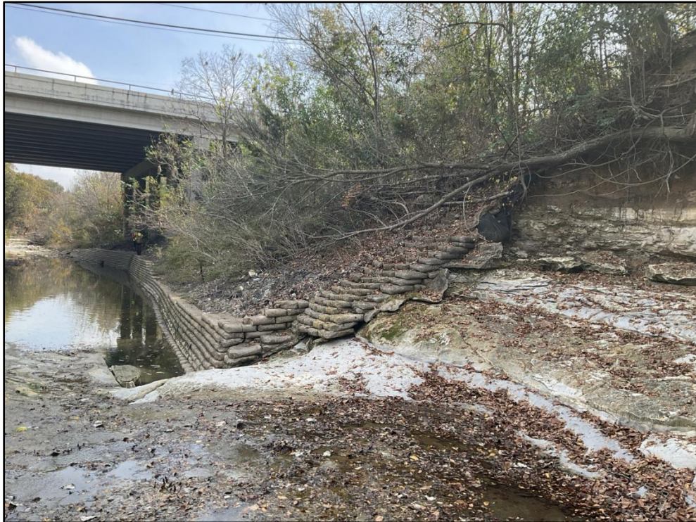
Photo 93 – Near STA 66+00 – Looking downstream at a concrete bag wall at South Cockrell Hill Road. Bag wall in fair condition, with some erosion at the upstream end and a trench in the channel bed along to toe.
