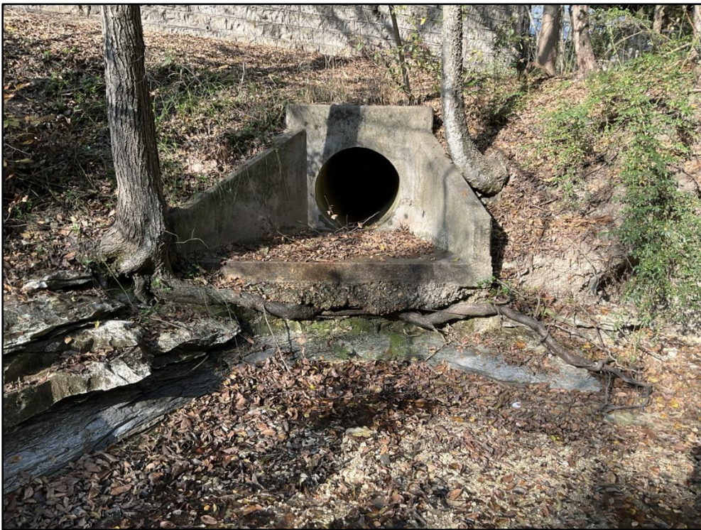
Photo 14 – Near STA 12+00 – Problem area rank: 15 . 30-inch concrete stormwater outfall on right bank. Flow line is approximately 28 inches above bed elevation.
