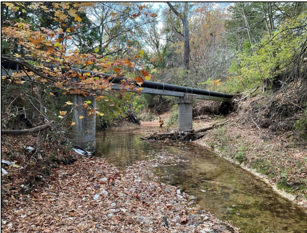
Photo 42 – Near STA 51+50 – Problem area rank: 5 (★ Area 2 ★) . Looking downstream at an 18-inch aerial sanitary sewer crossing. Significant scour on the right bank.
