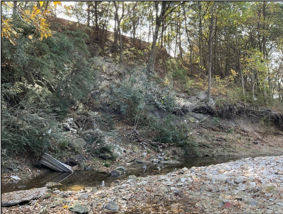
Photo 23 – STA 26+00 – Looking downstream, left bank is tall and steep. At this location, geotechnical bank failure is of greater concern than stream bank erosion.
