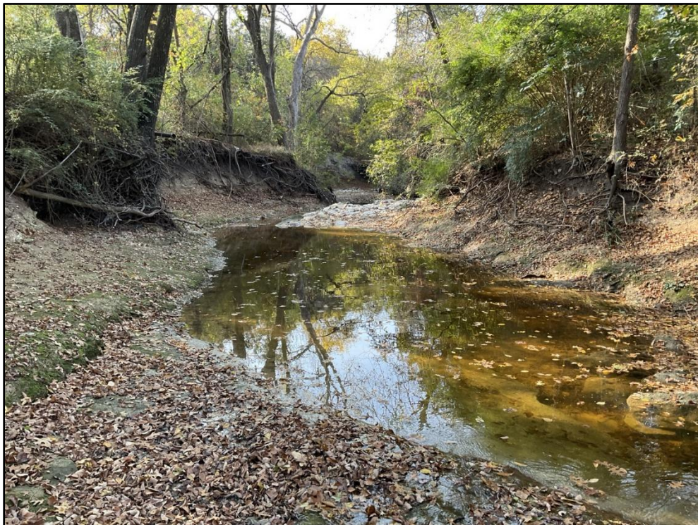
Photo 18 – Near STA 21+50 – Looking downstream. Left bank exhibits “High” BEHI rating.
